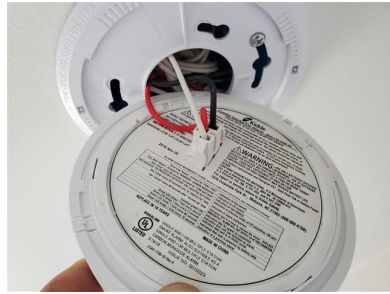
Hallway Combination Smoke and Carbon Monoxide Detectors (Hard-Wired/ Interconnected/ MFR Date 2016)
