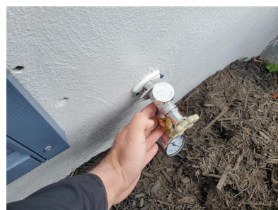
10.8 Item 1 (Picture) Hose Faucet Not Properly Secured (Front)
