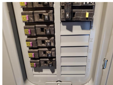
Space Available for Additional Circuits (Main Panel)
