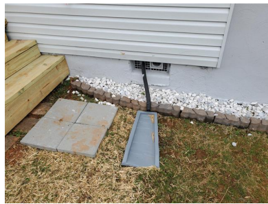
Crawl Space Sump Pump Discharge Location (Rear)
