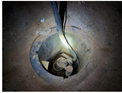
Crawl Space Sump Pump (Submersible/ See Comments)
