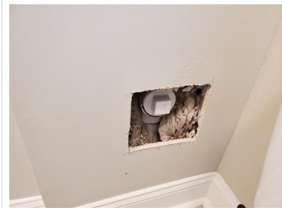
Waste Pipes (PVC/ Clean-Out Basement Bathroom Access Panel)
