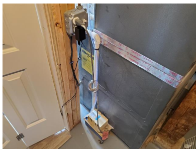
Condensate Drain and Pump (See Comments)
