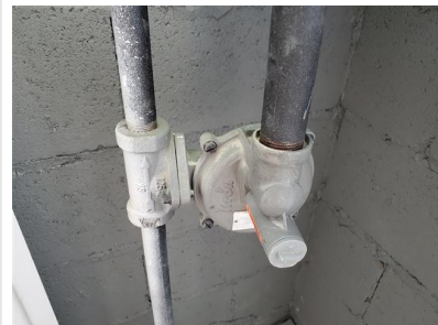
Gas Service Pressure Regulator (Meter)
