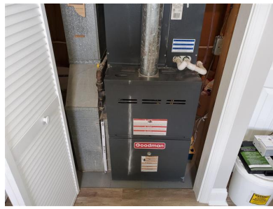
Furnace (Goodman/ Basement Utility Closet)
