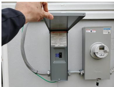
Electrical Service Emergency Disconnect (Rear Left)
