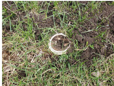
Sewer Line Clean-Out (Front Left/ Walk)
