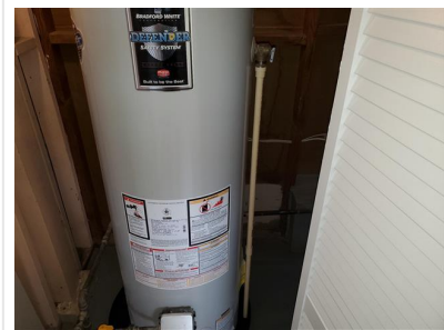
Water Heater Temperature and Pressure Relief Valve (Acceptable)
