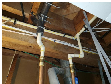
Distribution Pipes (CPVC)
