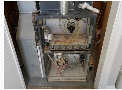
Furnace Service Covers Removed (A Little Dusty/ No Burned Wires/ No Condensate Leaks)
