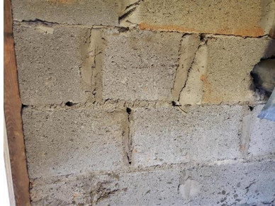
12.5 Item 2 (Picture) Drill Holes/ Previous Termite Treatment (Crawl Space Concrete Blocks)
