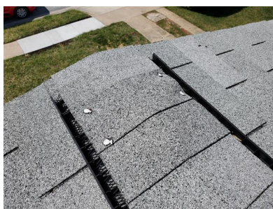
3.0 Item 4 (Picture) Improperly Sealed/ Exposed Nail Heads (Ridge Vents)
