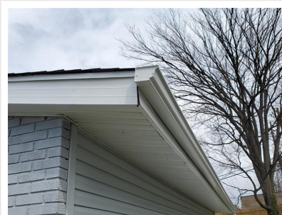
2.4 Item 1 (Picture) Gap/ Trim (Right Front Fascia Trim)
