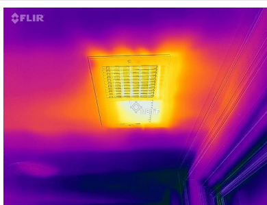
Furnace Supply Temperature (118°F)
