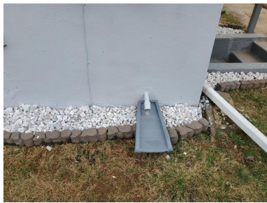
Basement Sump Pump Discharge Location (Rear Left)
