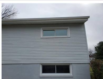
2.7 Item 1 (Picture) Screen Missing (Left Front/ Second Floor Window)
