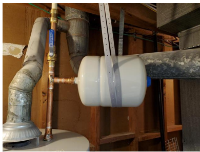
Water Heater Expansion Tank (Properly Supported)
