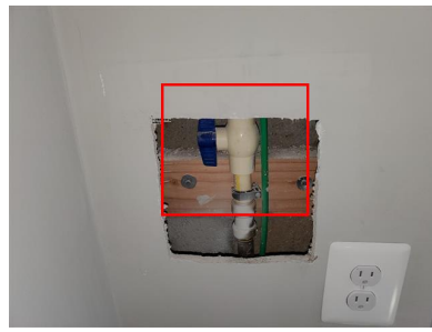
Water Service Main Shut-Off Valve (Basement Family Room/ Front Lower Access Panel)
