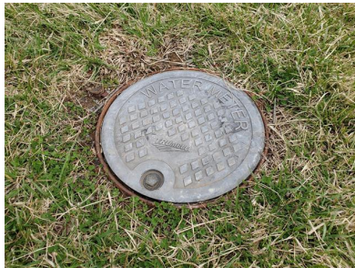
Water Service Meter (Front/Walk)
