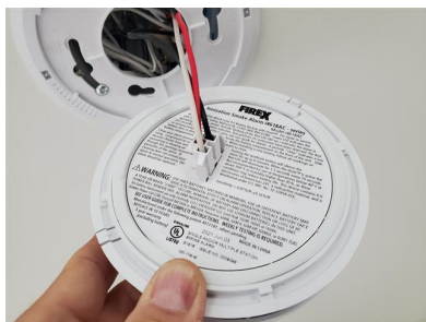
Bedroom Smoke Detectors (Hard-Wired/ Interconnected/ MFR Date 2021)
