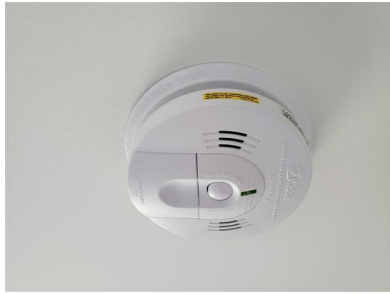
Hallway Combination Smoke and Carbon Monoxide Detectors (Acceptable)
