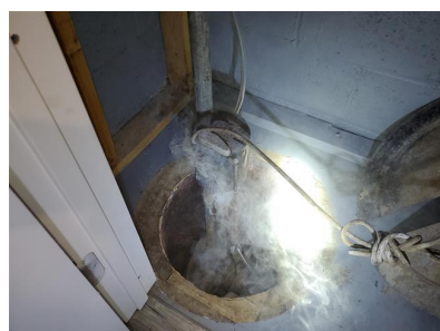
5.4 Item 2 (Picture) Sump Pump Damaged/ Inoperative (Basement Rear Left Closet/ Sump Pump 1)
