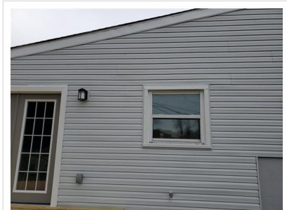
2.7 Item 3 (Picture) Screen Missing/ Damaged (Rear/ First Floor Window)
