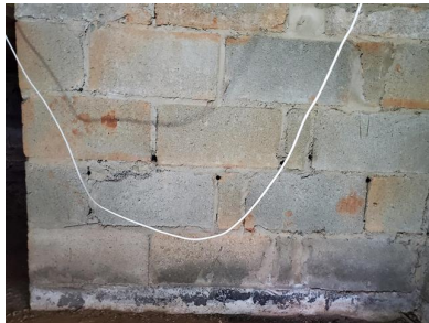
12.5 Item 3 (Picture) Drill Holes/ Previous Termite Treatment (Crawl Space Concrete Blocks)
