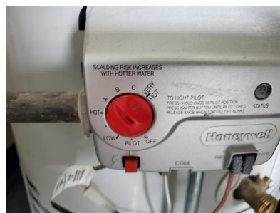
10.7 Item 3 (Picture) Thermostat Set High (Water Heater)
