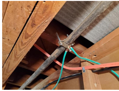
Electrical System Bonding (Gas Service Pipe)
