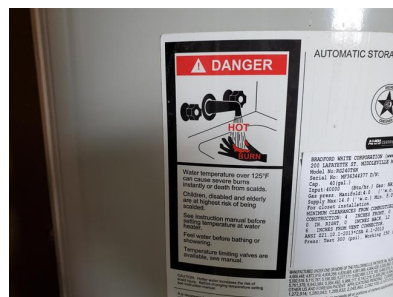
10.7 Item 4 (Picture) High Water Temperature Warning (Water Heater)
