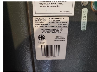
Evaporator Coil Data Tag (MFR Date 2013/ 3.0 Ton)
