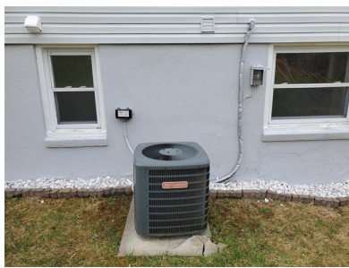
Central AC Condenser (Goodman/ Rear)
