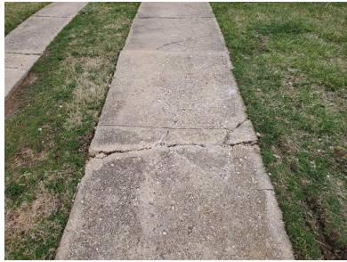
2.0 Item 1 (Picture) Driveway Deteriorated (Front Left)
