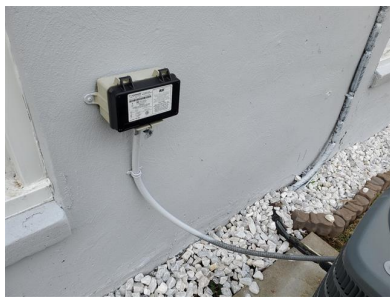
BGE Peak Rewards Energy Savings Program Cycling Meter (Contact Utility to Transfer Service)
