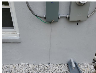
Electrical System Grounding (Driven Rod/ Rear Left)
