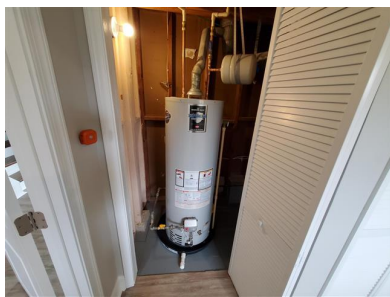
Water Heater (Bradford White/ Natural Gas/ Basement Utility Closet)
