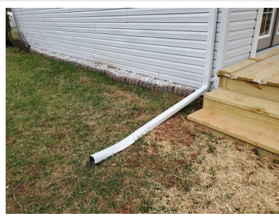
5.0 Item 1 (Picture) Downspout Extension Crushed (Rear Right Downspout)
