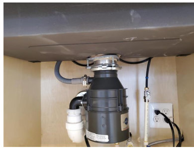
Dishwasher Drain Line High Loop Present (Good/ Kitchen Under Sink)
