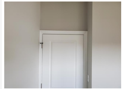
7.6 Item 3 (Picture) Door Binding (Second Floor/ Left Front Bedroom)
