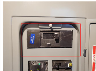
Electrical Service Main Disconnect (Main Panel)
