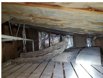
Attic Insulation (Fiberglass Batts/ 4 Inches)
