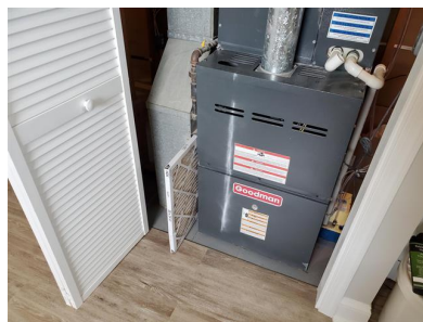
Air Filter Location (Basement Utility Closet/ Furnace)
