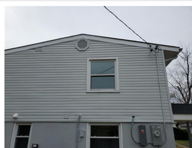
2.7 Item 2 (Picture) Screen Missing/ Damaged (Rear Left/ Second Floor Window)
