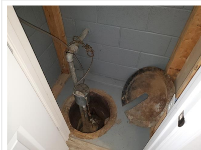
5.4 Item 3 (Picture) Battery Back-Up System Not Present (Basement Sump Pump)
