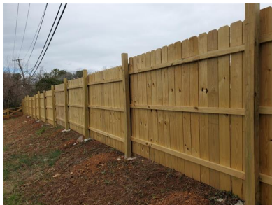
2.12 Item 3 (Picture) Fence Post Caps Missing (Rear Fence)
