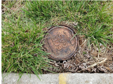
Gas Service Shut-Off Valve/ Street (Front Left)
