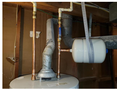
Water Heater Exhaust Flue (Acceptable/ Combination Vented with Furnace)
