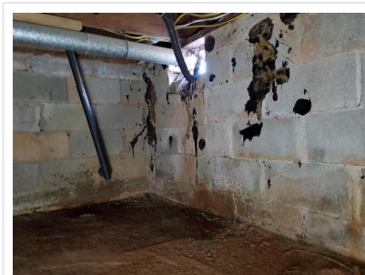
5.4 Item 5 (Picture) Discharge Line Leaks When Pump Activated (Crawl Space Sump Pump)
