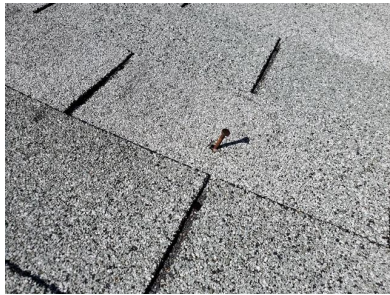
3.0 Item 1 (Picture) Partially driven/ Improperly Sealed Nail (Left Front Roof)
