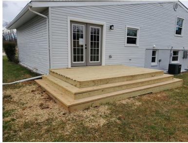
2.12 Item 2 (Picture) Deck Bare/ Not Painted or Stained (Rear)
