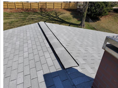
Attic Ventilation (Ridge Vents)
