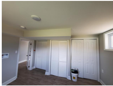
9.4 Item 2 (Picture) Supply Registers Missing (Basement Laundry Room)
