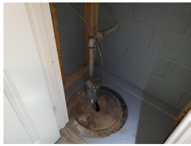
Basement Sump Pump (Rear Left Closet)
