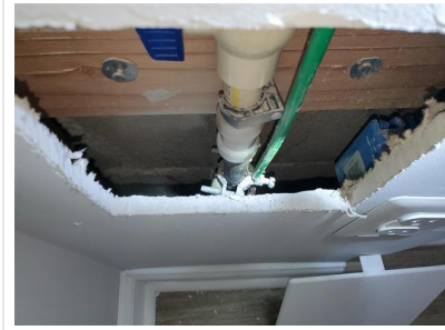
Electrical System Grounding/ Bonding (Water Service Pipe)
