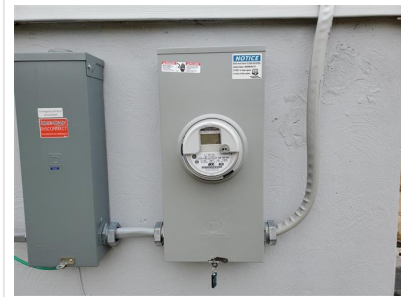
Electrical Service Meter (BGE/ 200 Amp/ Properly Secured)
