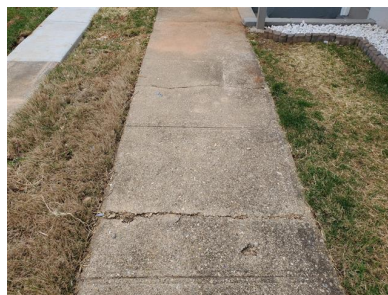
2.0 Item 6 (Picture) Driveway Cracked (Multiple Locations)
