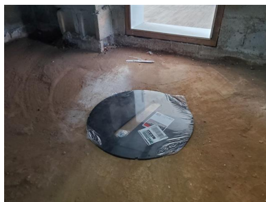
5.4 Item 8 (Picture) Cover Not Installed (Crawl Space Sump Pump)
