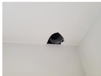
13.7 Item 1 (Picture) Clothes Dryer Vent Does Not Extend Below Ceiling (Basement Laundry Area)
