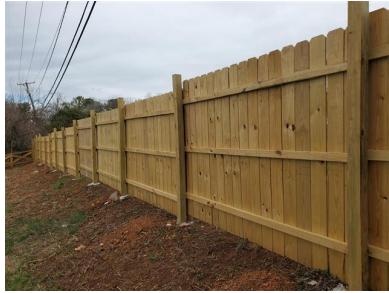
2.12 Item 1 (Picture) Fence Bare/ Not Painted or Stained (Rear)
