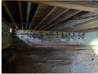
6.3 Item 2 (Picture) Insulation Missing (Crawl Space/ Foundation Walls)
