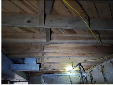
6.3 Item 1 (Picture) Insulation Missing (Crawl Space/ Between Floor Joists)
