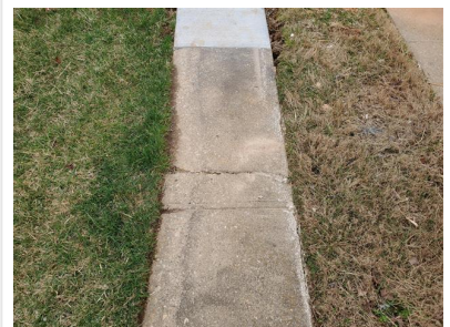
2.0 Item 7 (Picture) Driveway Cracked (Multiple Locations)
