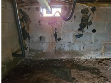
12.5 Item 1 (Picture) Drill Holes/ Previous Termite Treatment (Crawl Space Concrete Blocks)
