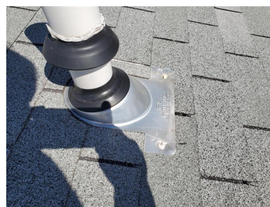
3.0 Item 5 (Picture) Improperly Sealed/ Exposed Nail Heads (Plumbing Stack Vent Flashing)
