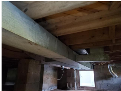
9.4 Item 3 (Picture) Insulation Missing (HVAC Ductwork/ Crawl Space)
