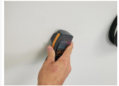
7.2 Item 3 (Picture) Moisture Meter Confirmed Wet Conditions (Front Left Bedroom)
