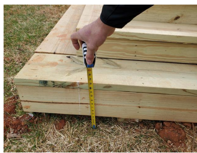
2.8 Item 2 (Picture) Lower Step Riser Height Excessive (Rear Deck)
