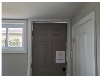
2.6 Item 1 (Picture) Door Binding (Left Rear Basement Entrance Door)
