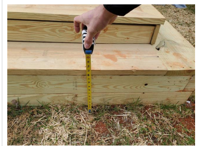
2.8 Item 3 (Picture) Lower Step Riser Height Excessive (Rear Deck)
