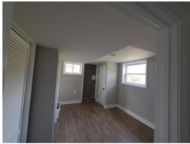
9.4 Item 1 (Picture) Supply Registers Missing (Basement Laundry Room)
