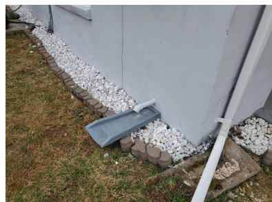
5.4 Item 1 (Picture) Sump Pump Discharges Too Close to Foundation (Rear Left)
