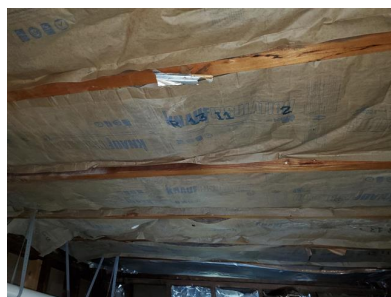
Attic Insulation (Fiberglass Batts/ 4 Inches)
