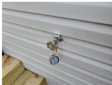
Rear Hose Faucet (Properly Secured)
