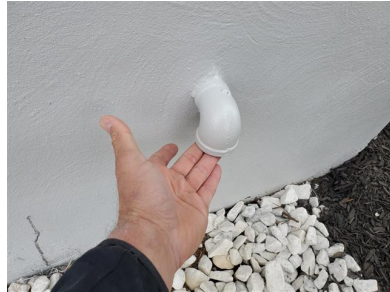
Gas Service Vent (Screened/ Left Front)
