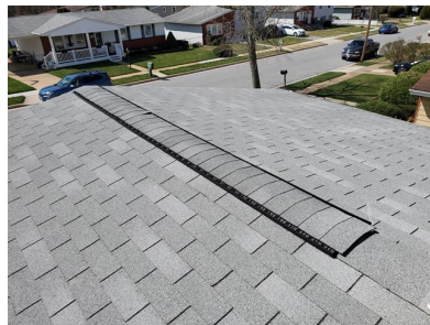
Attic Ventilation (Ridge Vents)
