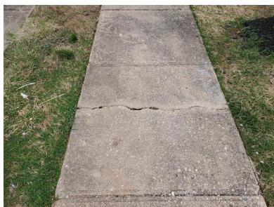
2.0 Item 5 (Picture) Driveway Cracked (Multiple Locations)
