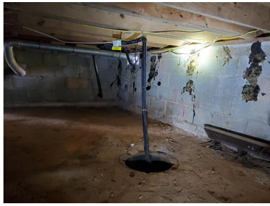
Crawl Space Sump Pump (Crawl Space/ Rear)
