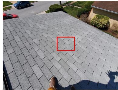
3.0 Item 2 (Picture) Partially Driven/ Improperly Sealed Nail (Left Front Roof)
