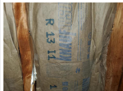
Attic Insulation (R-13 Value)
