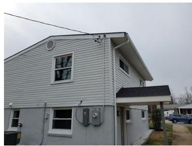
Electrical Service Entrance (Rear Left)
