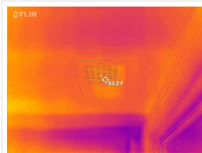
9.1 Item 3 (Picture) Cooling System Supply Temperature (63°F)
