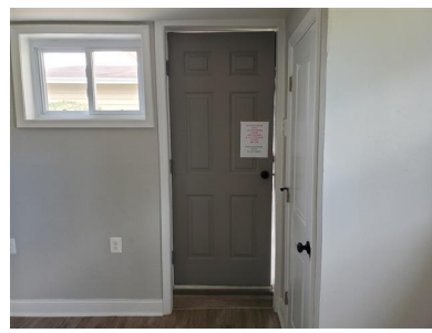
2.6 Item 2 (Picture) Door Binding Perspective Photo (Left Rear Basement Entrance Door)
