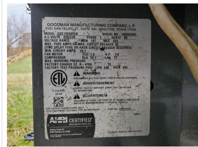
Condenser Data Tag (MFR Date 2014/ 3.0 Ton/ Refrigerant R-410A)
