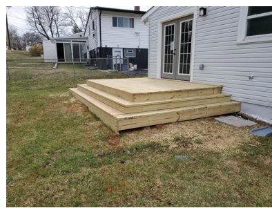
2.8 Item 1 (Picture) Lower Step Riser Height Excessive (Rear Deck)
