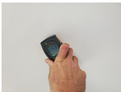
7.2 Item 4 (Picture) Moisture Meter Control Reading (Front Left Bedroom)
