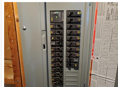
AFCI/ GFCI Resets (Main Panel)
