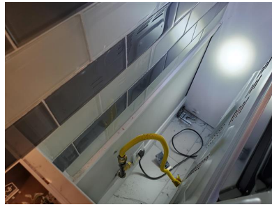
Anti-Tip Bracket Installed (Good/ Kitchen Range/ Oven)
