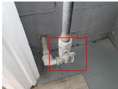
Gas Service Main Shut-Off Valve (Meter)
