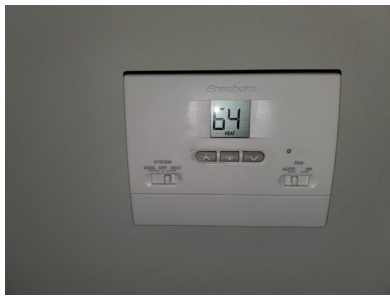
Thermostat (First Floor Dining Room/ Interior Wall)
