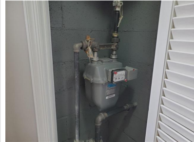
Natural Gas Meter (Basement Front Left Closet)
